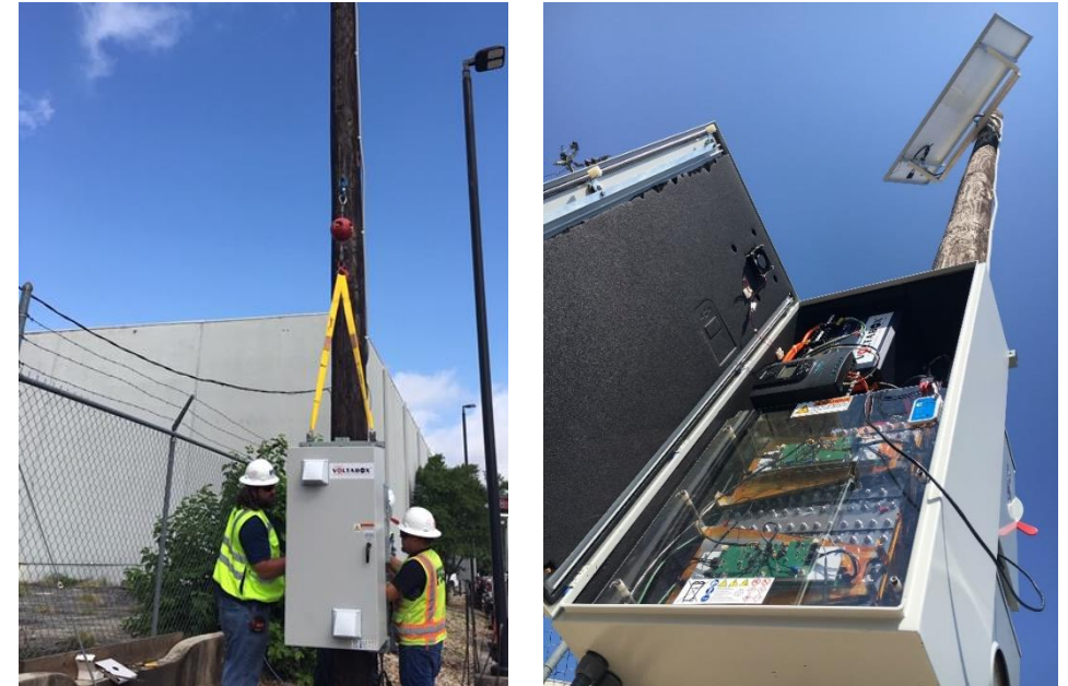
Images: Prototype installations of the Voltabox systems in Austin/TX
